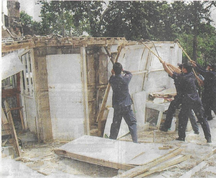
Tear it down: Enforcement officers demolishing a structure at a former site of the Ajaran Banuar movement in Meru.
