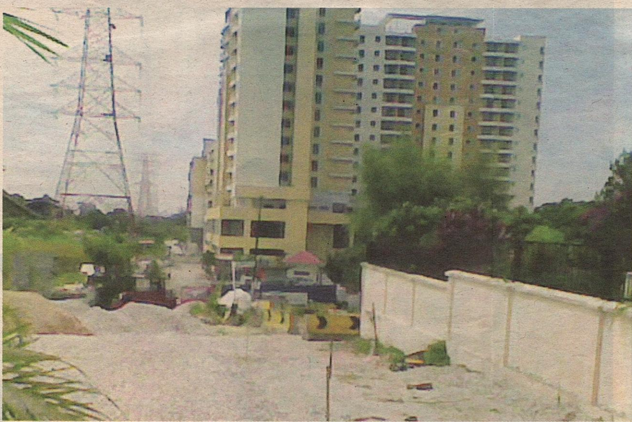
SOON TO BE COMPLETED: The Paramount View Condo project in Taman Aman. Note the distance between the wall of the house on the right and the worksite
