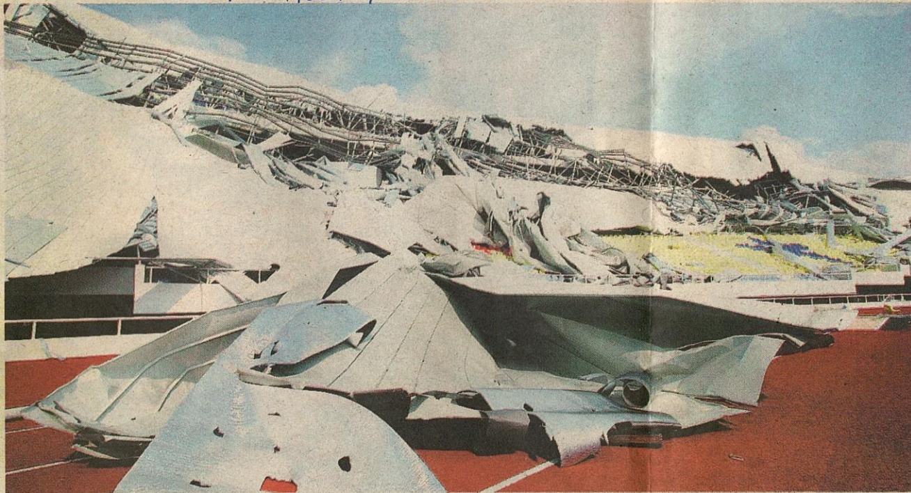
About 60 per cent of the roof of the Sultan Mizan Zainal Abidin Stadium collapsed at 9.30am on Tuesday. — Bernama picture
