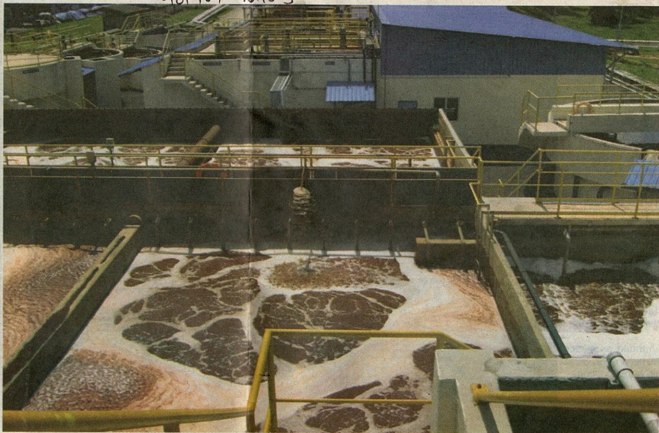
A Storm Water Treatment Plant treats 600 cubic metres of contaminated rainwater daily. The treated storm water is rechannelled to the various plants for use to conserve waste usage.
