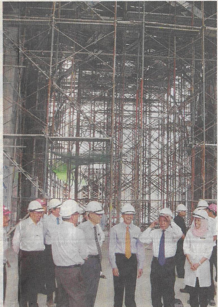
Getting ready: Raja Nong Chik (in orange tie) sharing a light moment with Samsudin as the latter adjusts his hard hat before a tour of the City Mosque.
