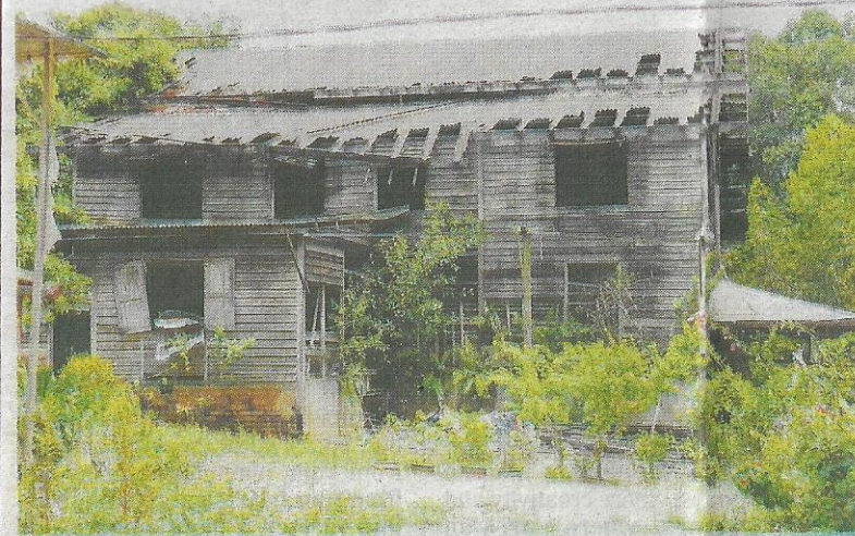
The dilapidated old smokehouse at the village.
