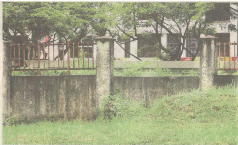
Missing: Illegal scrap metal collectors often steal grilles in public areas.
