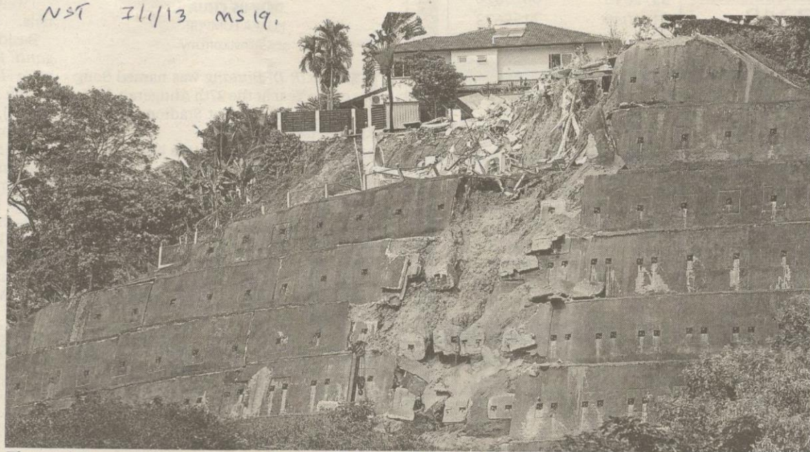
The retaining wall that collapsed in Puncak Setiawangsa on Dec 28.
