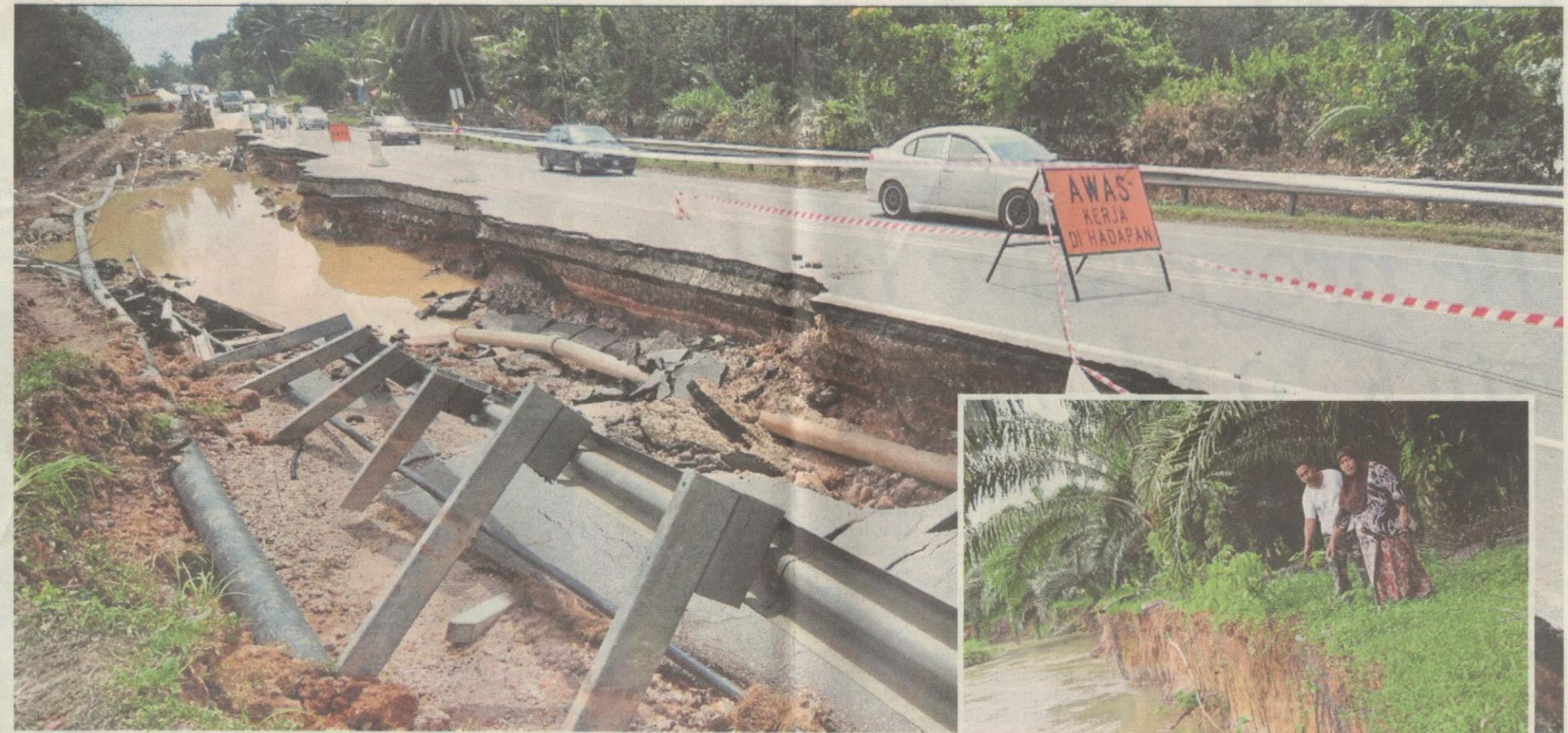
Soil erosion during the recent monsoon season damaged roads and riverbanks, such as the Jerantut-Temerloh road in Pahang and the rivers near villages in Kulim, Kedah (inset). To alleviate the problem, we need to reduce the impact of water on soil as well as increase the ability of the soil to resist erosion .
