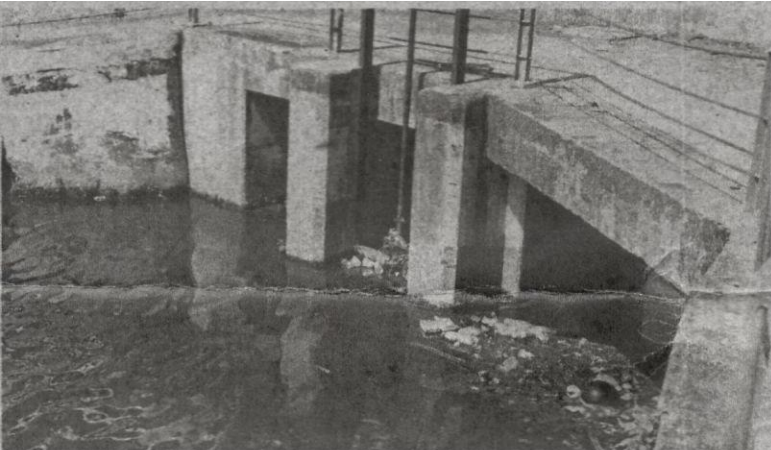
Stakeholders want MBPJ to remove drainage connectivity from the surrounding neighbourhoods into the lake in Taman Jaya.
