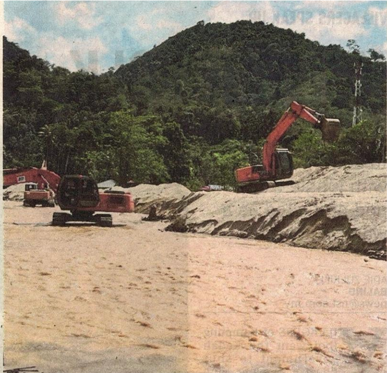
Excavators removing sand and mud in Sungai Kupang, Baling, recently. PIX BY ADIE ZULKIFLI
